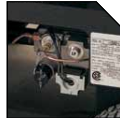
LP-gas shut-off valve
